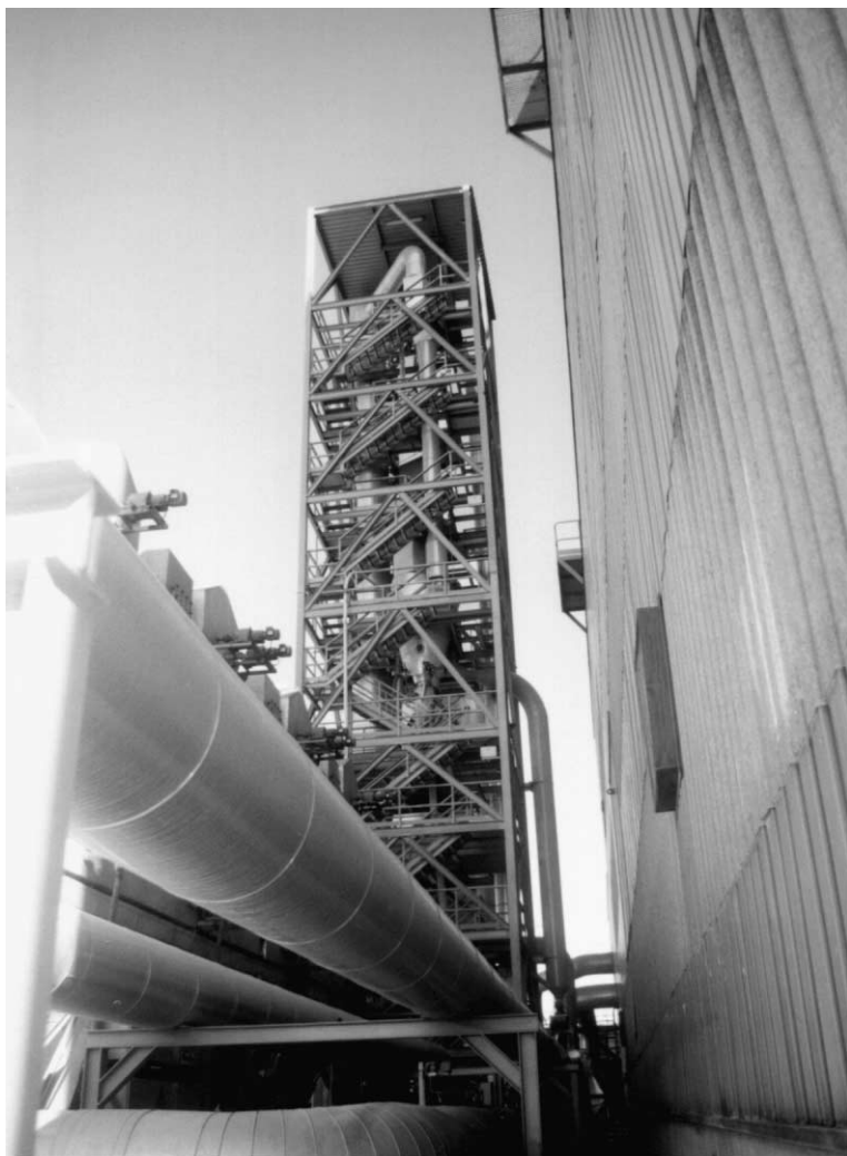
Fig. 2. View of the Los Barrios pilot plant.
